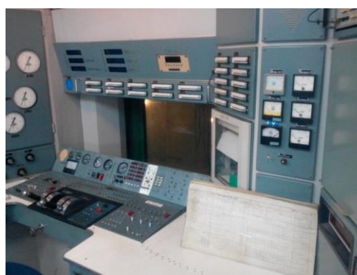
Fig. 5. Operator control panel
