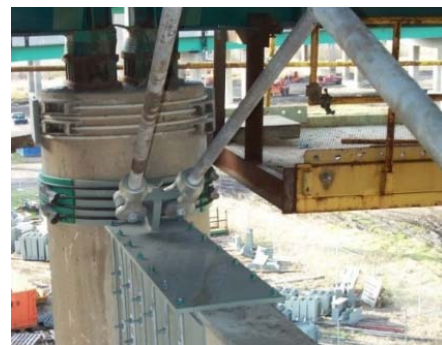
Fig. 8. General view of "flat-jack" support
