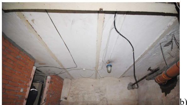
Fig.1. a), b) Floor slab in the form of vaults over the steel beams [5]
